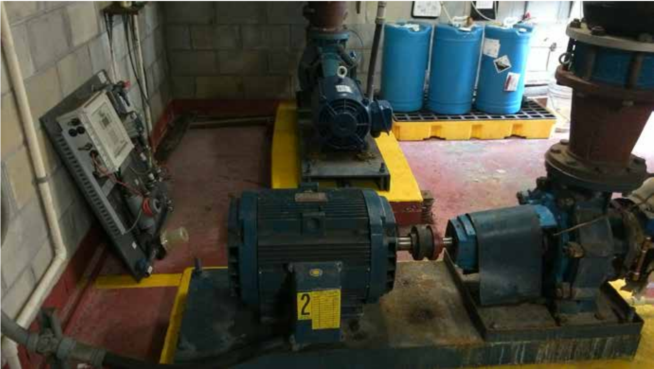
A/C Circulating Pumps
