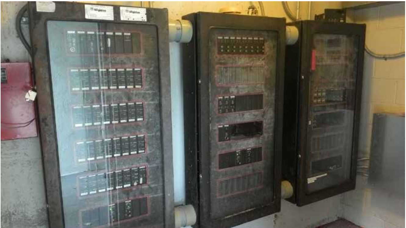
Fire Alarm Panel
