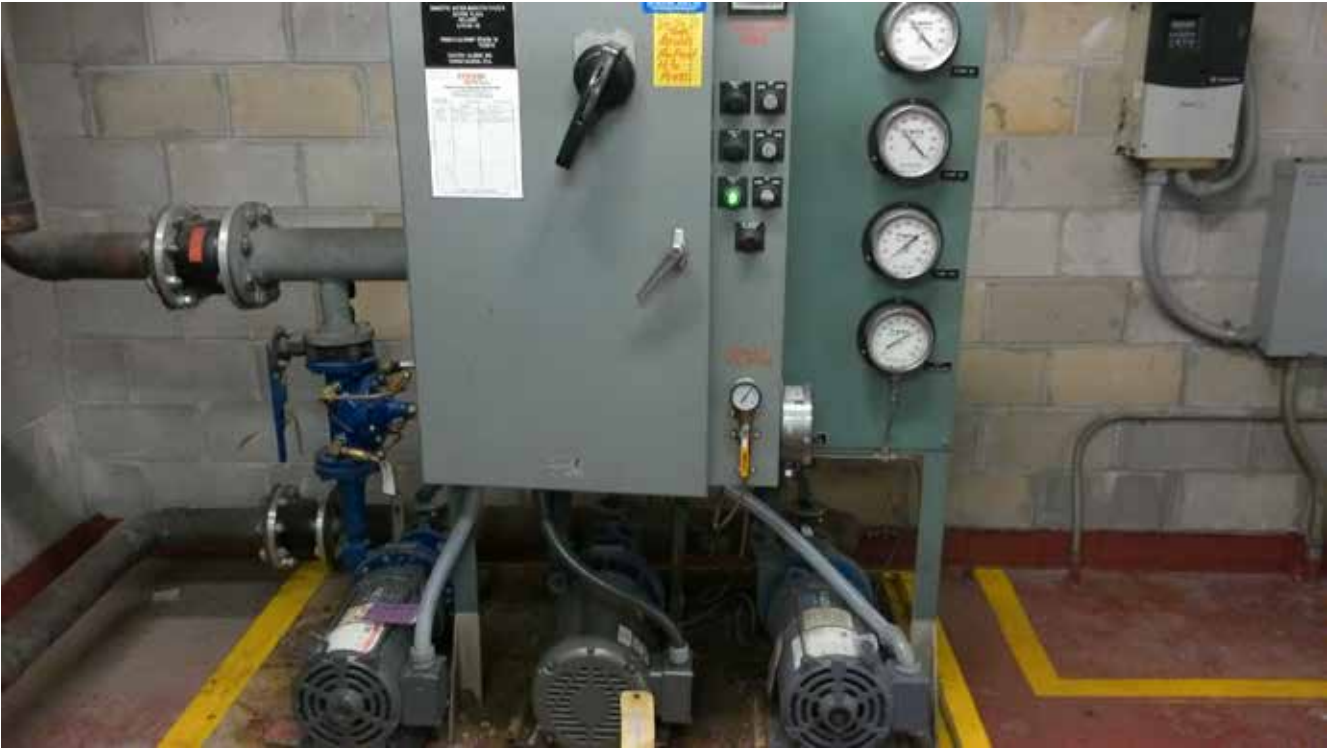
Domestic Water Pumps
