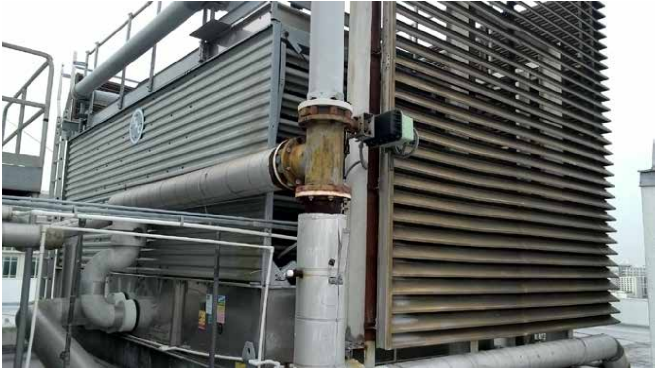
A/C Cooling Tower
